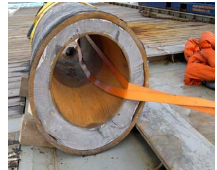
Cut and retrieved Conductor stub
